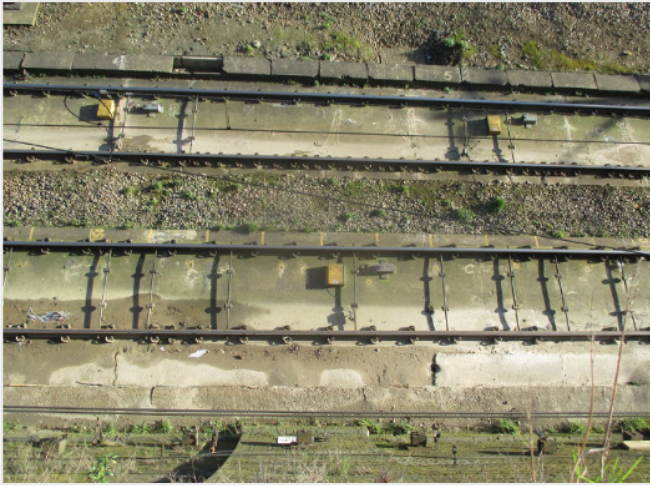
Figure 11: Cracking on Kentish Town slab track.
