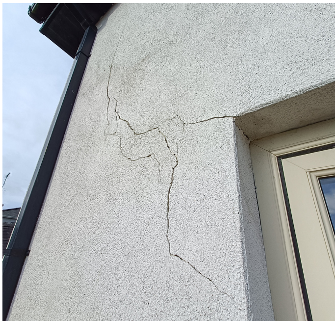
Cracks in plaster
