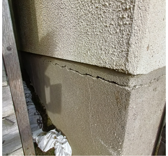
Crack in exterior
